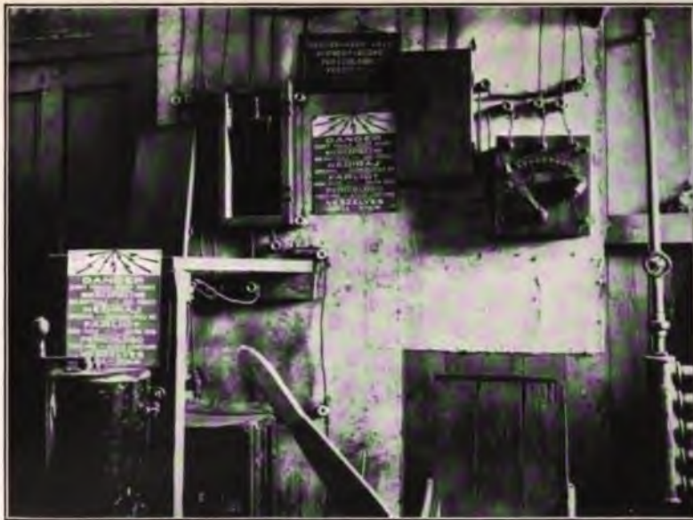
PLATE 14.—MILL SWITCH BOARD SHOWING METHOD OF MARKING ELECTRICAL EQUIPMENT
